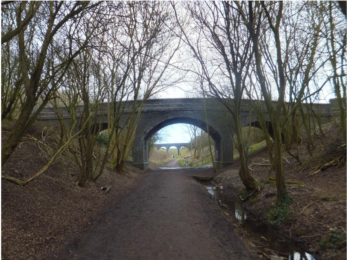
Figure 12 Looking northeast along the GCR trackbed with a footbridge visible ahead of Newton Lane road bridge (SP 5286 7838).
