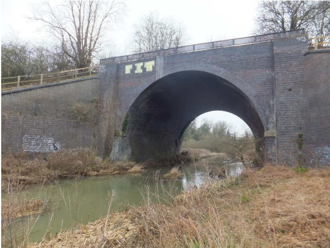
Figure 5 Looking west at the bridge carrying the GCR trackbed over the River Avon (SP 5180 7652).
