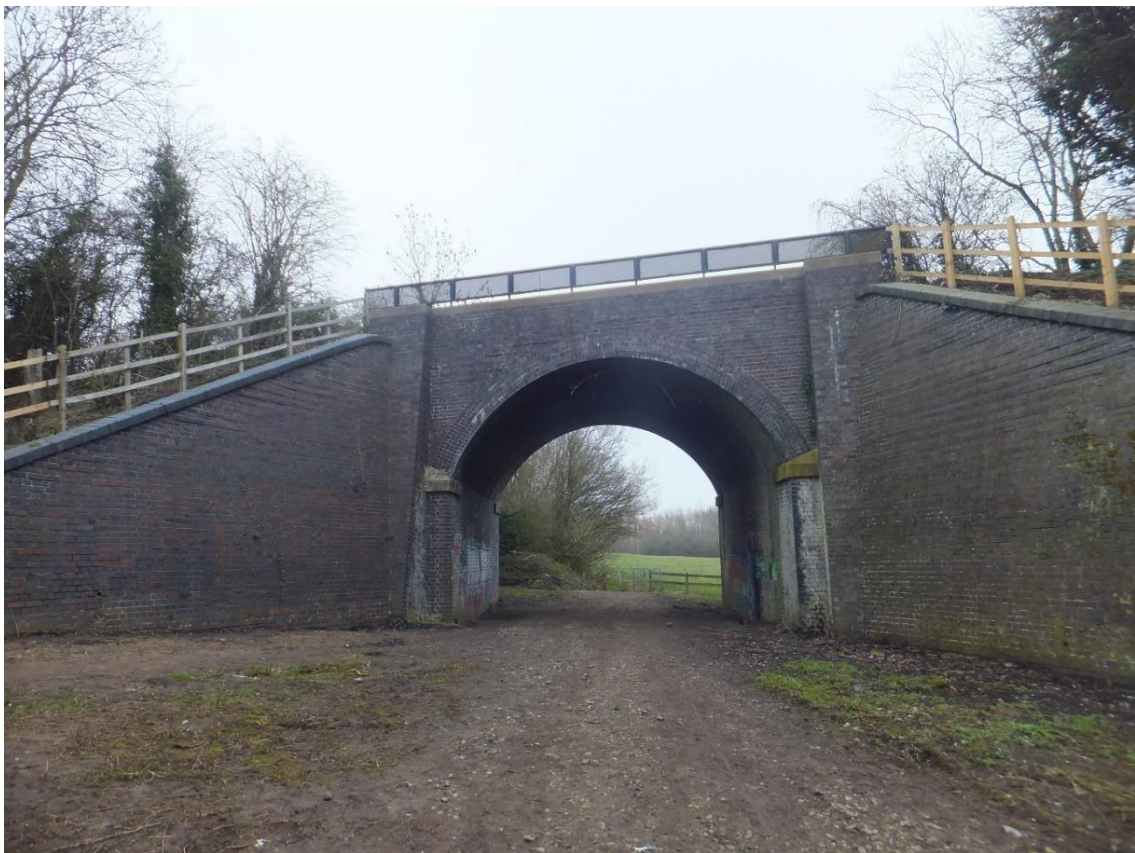
Figure 6 Looking west at the bridge carrying the GCR trackbed over a footpath between Rugby and Clifton upon Dunsmore (SP 5183 7666).
