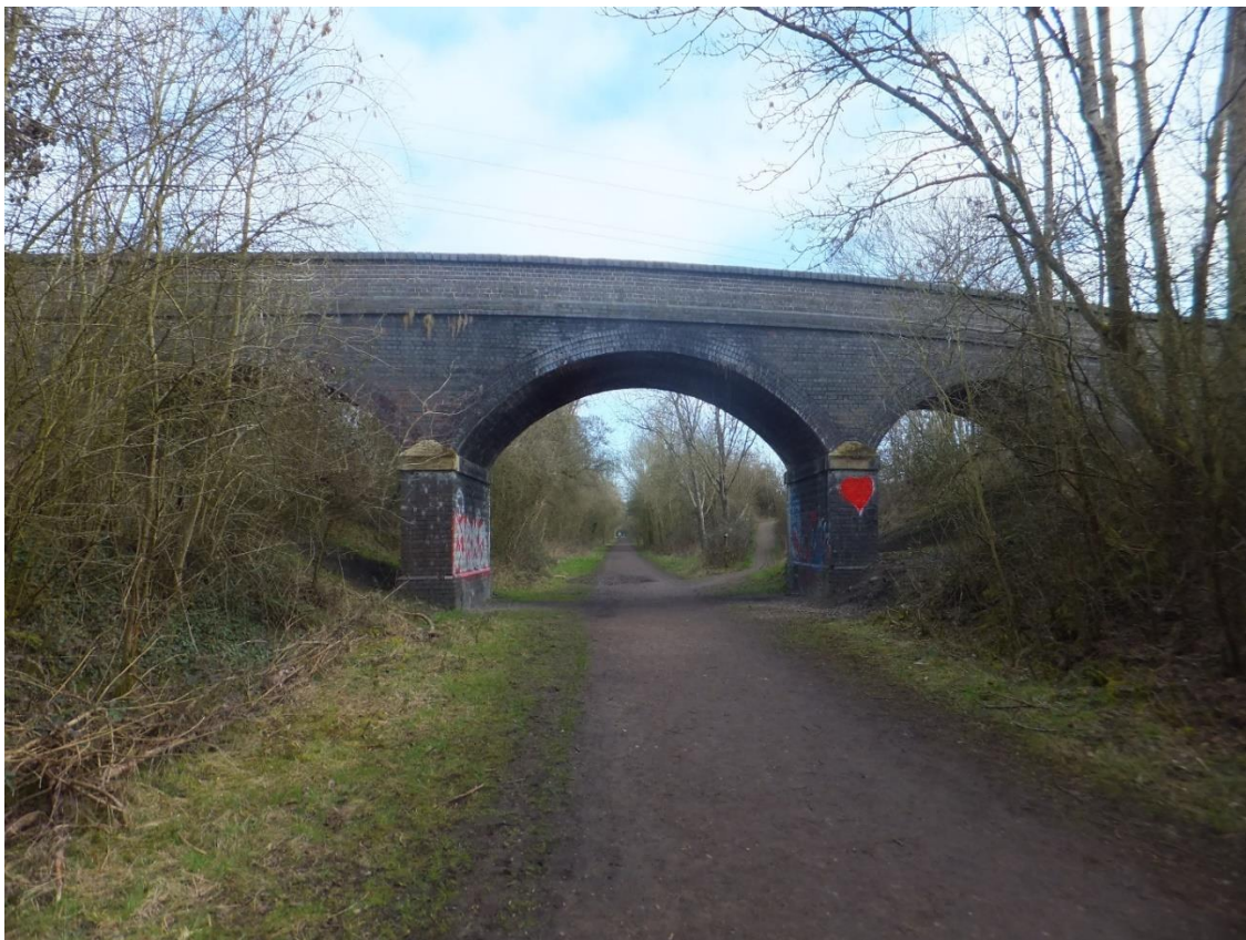
Figure 10 Looking northeast along the GCR trackbed where the bridge to Newton House Farm crosses (SP 5252 7791).
