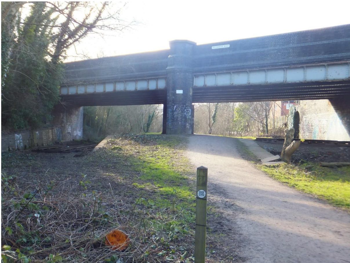
Figure 10 Looking south at Hillmorton Road bridge and the northern extent of the Rugby Central station platform (SP 5137 7467).
