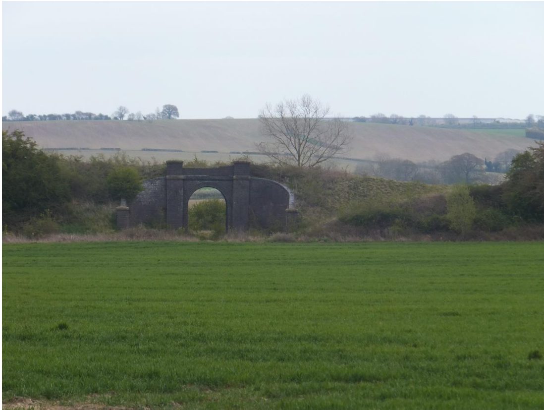
Figure 16 Close-up looking east at the farm access point within the GCR embankment, showing how the height of the embankment has been reduced to the right of the bridge (SP 5244 6478).
