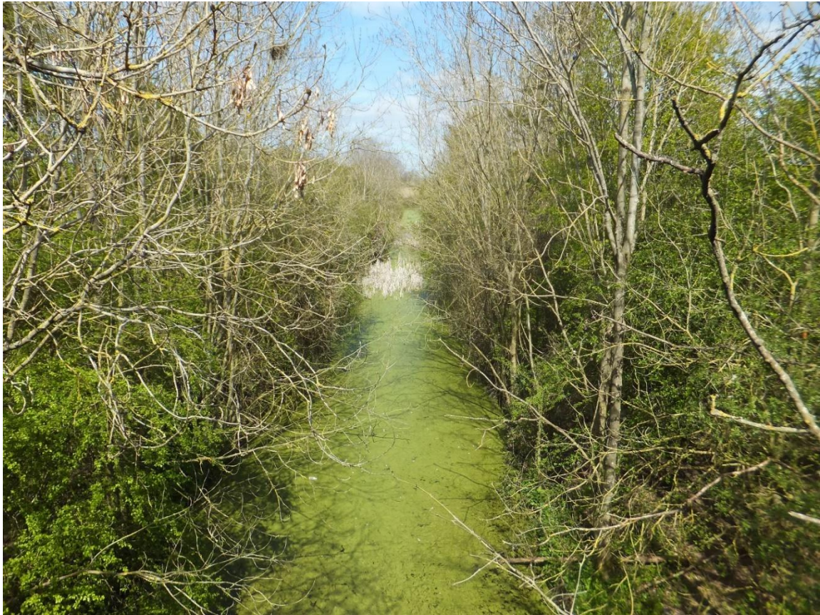
Figure 11 Looking north from the overbridge at the water-filled trackbed near Flecknoe (SP 5238 6354).
