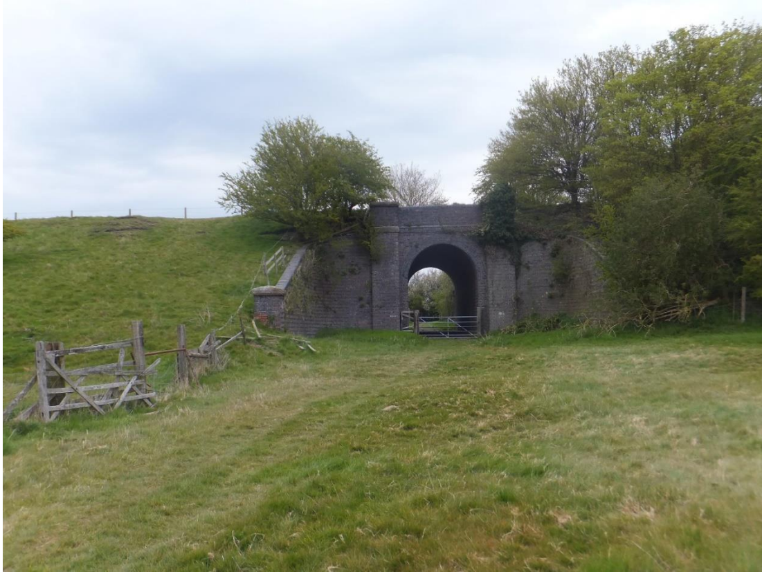
Figure 23 The access bridge within the GCR embankment where the marked bridleway passes through it, south of Willoughby (SP 5242 6637).
