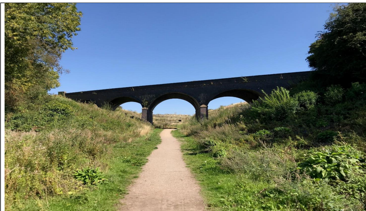
Caption Above: Newton Lane Bridge. The old Great Central was designed to a generous loading gauge and standard clearance of bridges. If the Great Central and feeder links are rebuilt, these could be made to continental loading gauge to enable things like an inland roll-on, roll-off rail network to cart vehicles across the country and things like a spinal railway distributor corridor to offer Piggyback could be nurtured. Picture by Mr Stephen Byatt 2018
